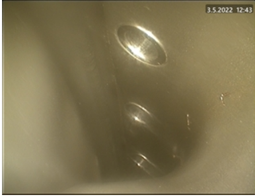
Burner #14_ring channel (1)
