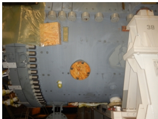
RHS turbine side
