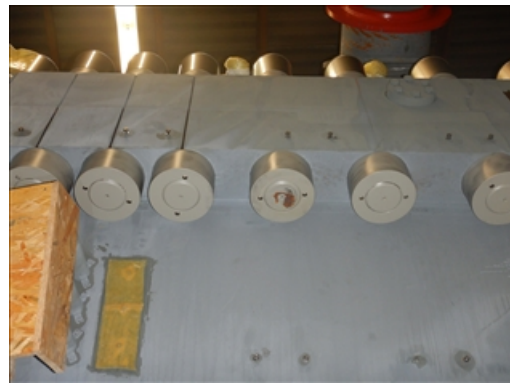
turbine side half joint bolt (1)
