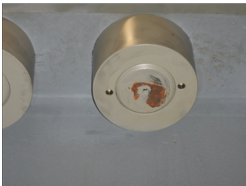
turbine side half joint bolt (2)
