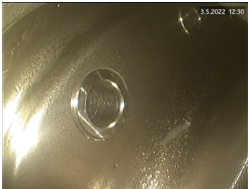
Burner #10_inner channel (1)
