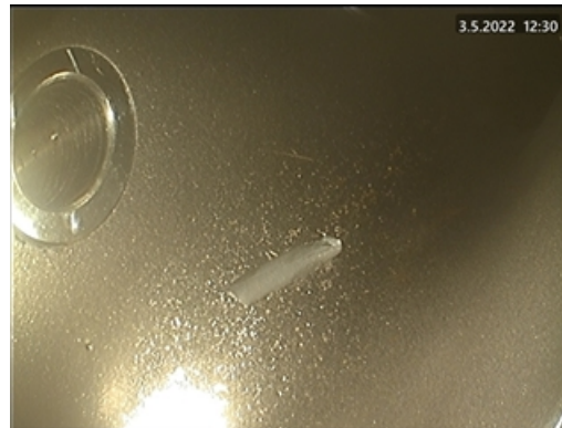
Burner #10_inner channel (2)
