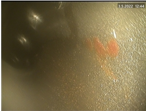
Burner #14_ring channel (3)
