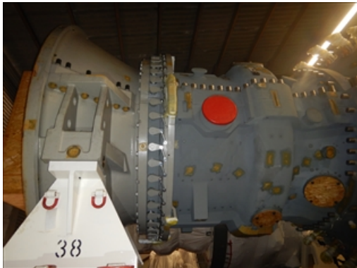
RHS compressor side (1)
