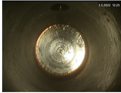
Burner #10_vane hole (1)
